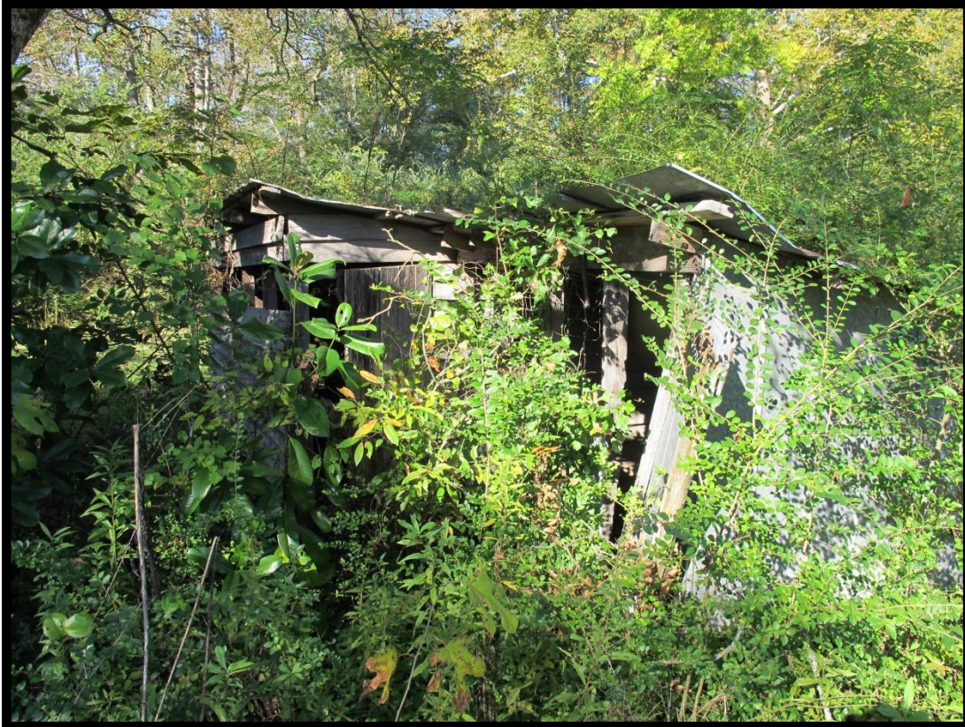
Figure 84: Frank D. Byrd House (# 041), Dilapidated Sheds Looking Northwest.
