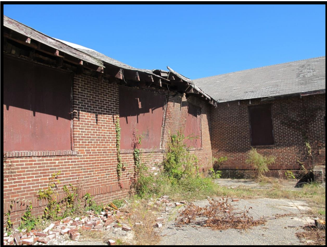
Figure 63: (Former) Bunnlevel Elementary School (# 026), Detail of Partially Collapsed Wall.
